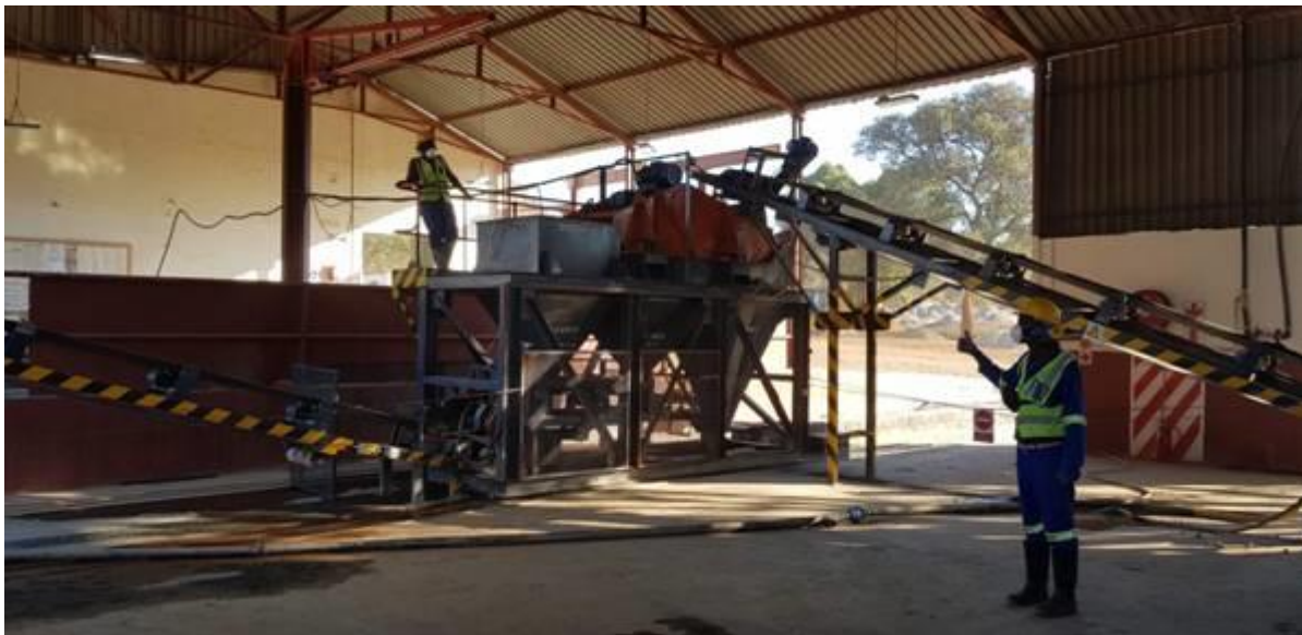
Figure 4. View of the completed screening and dewatering circuit of the processing plant.
