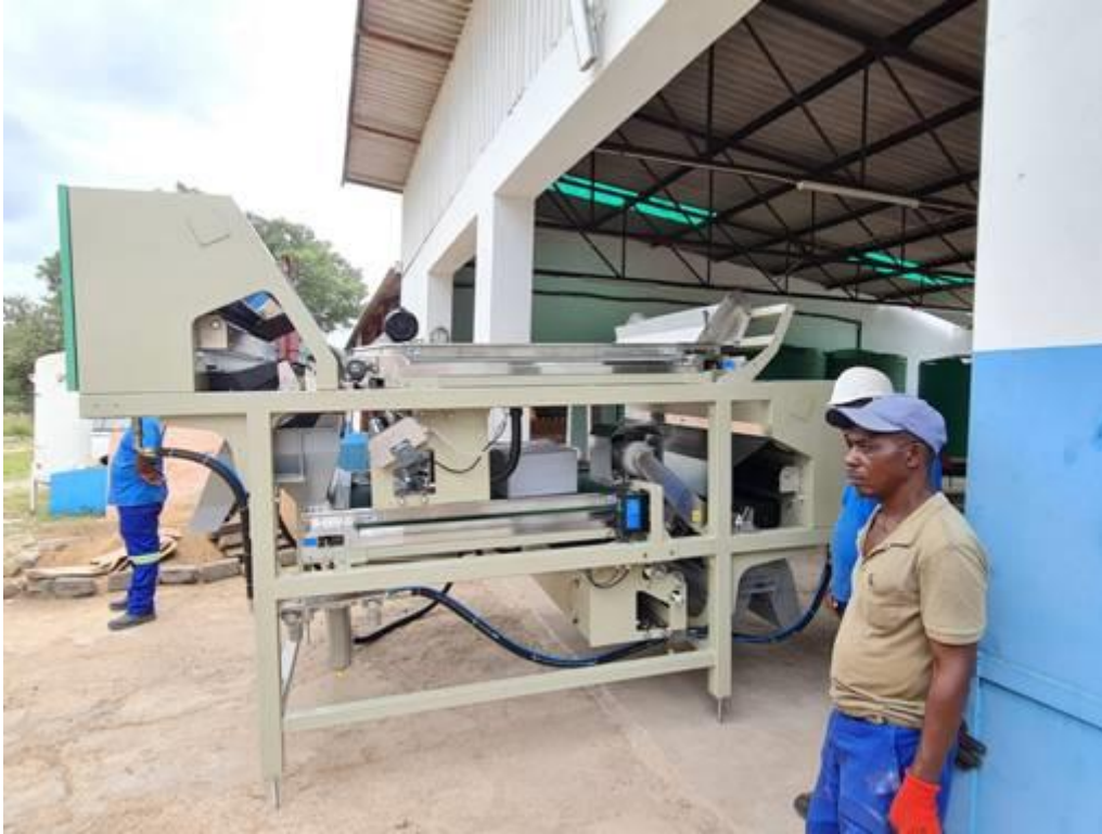
Figure 3. Main sorter unit offloaded in front of processing and sorting facility.
